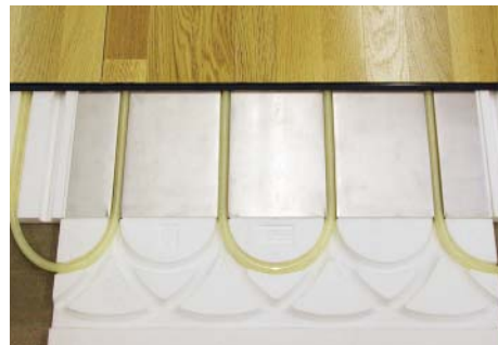
1B. Roth Radiant Panel System on slab
